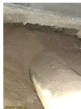
Construction gap crawlspace
