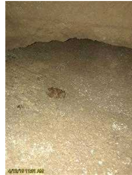
Construction gap crawlspace
