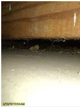
Construction gap 5 feet
