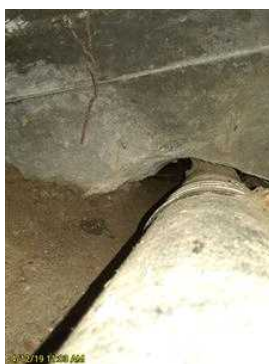
Construction gap crawlspace
